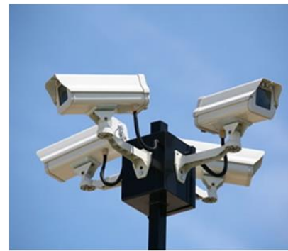
Improved security with CCTVs to record operations
